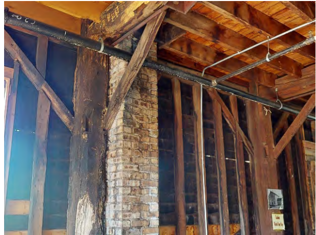
Second floor, missing bent members.
