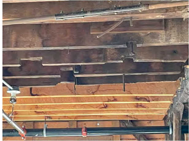
Compromised wood members supporting first floor.
